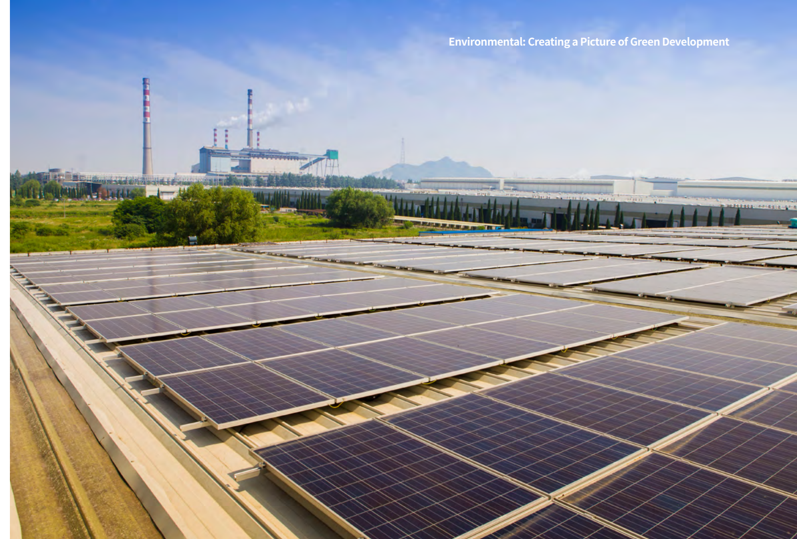
Gold East Paper's rooftop photovoltaic power project
